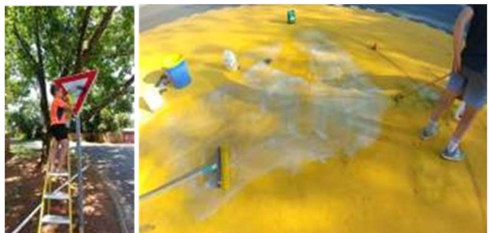
100's of Illegal Posters, Wires, & Cable Ties removed. As well as Graffiti.
